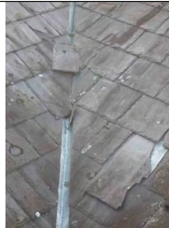
Fig.2: Slipped slate to the valley junction between the main block and the south wing.
