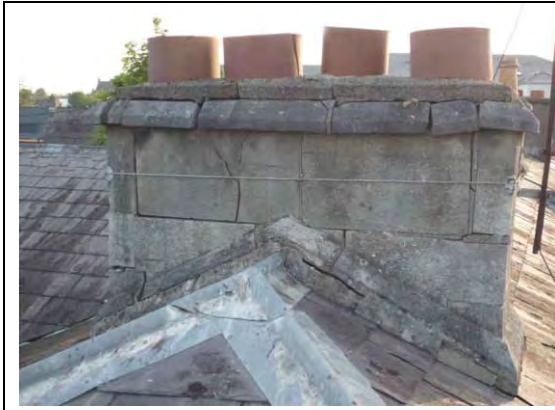
Fig.15: Fracturing of stonework to chimneys likely to have been caused by corrosion jacking of the masonry.
