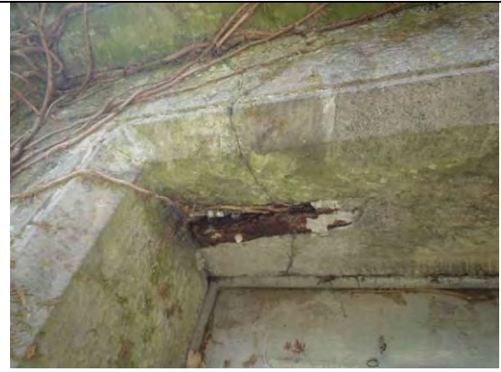
Fig.16: Fracturing of lintel to west door surround caused by corrosion jacking - note the exposed corroded metal cramp.
