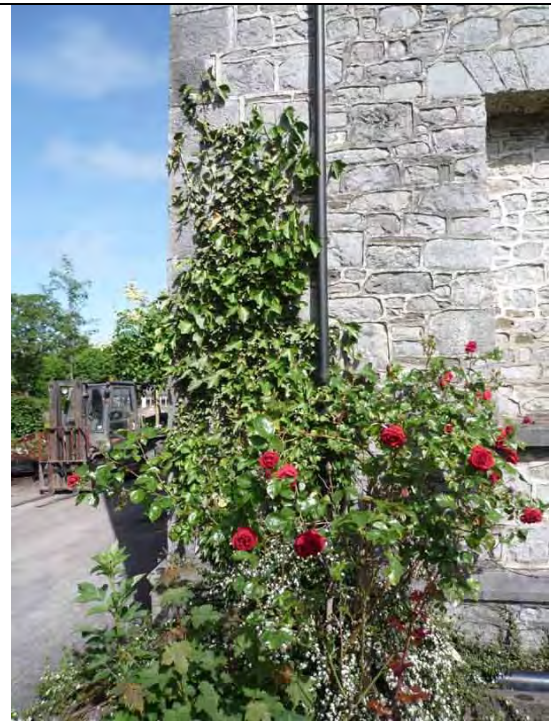
Fig.30: Ivy growth to the south elevation.
