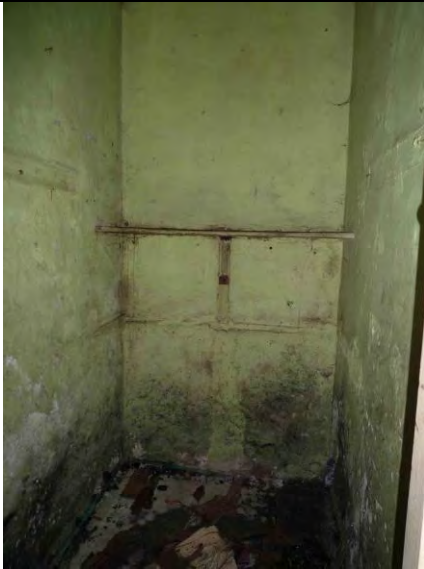
Fig.59: Plaster failure at low level as a result of rising damp to G20.
