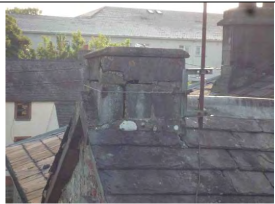
Fig.18: Fracturing of blocking course rising over the north pedimented breakfront.
