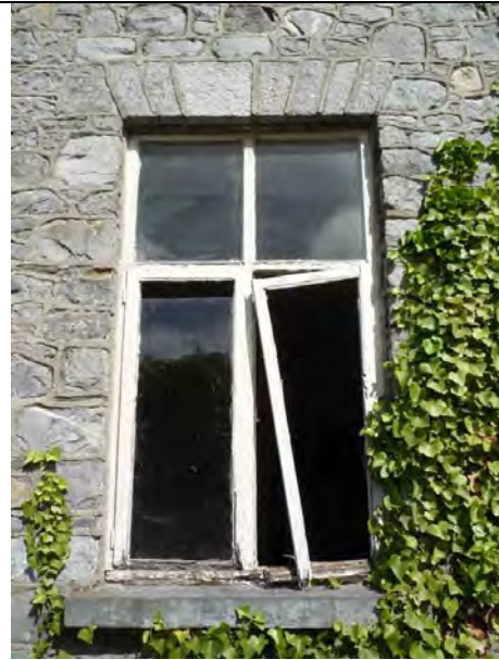
Fig.34: Complete failure of the timber casement windows.
