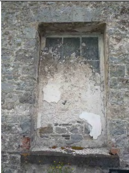
Fig.35: Blind window opening with trace remains of trompe-l'oeil window to ground floor (east) of north elevation.
