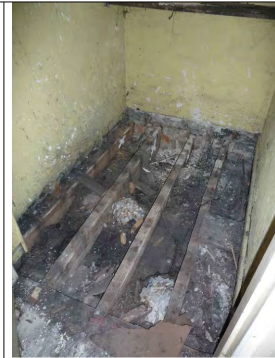
Fig.46: Missing floorboards to F06.
