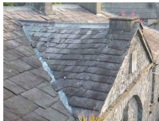
Fig.4: Deflection in the roofing plane of the south wing. Note the slipped slate as a result.
