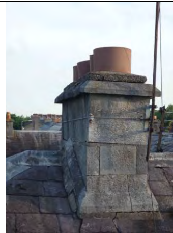
Fig.6: Cracked and failed mortar fillet to the base of chimney stacks.
