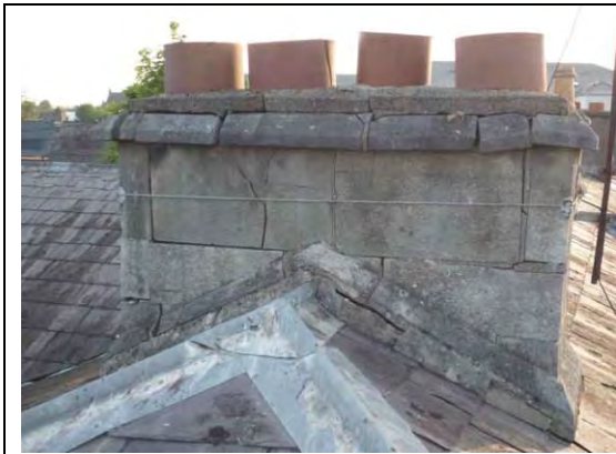
Fig.17: Significant fracturing of masonry to chimney stacks as a result of corrosion jacking.
