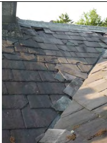
Fig.3: Notable failure of the roof to the north wing. Note the concentration of slipped slates and hole exposing roofing timbers.
