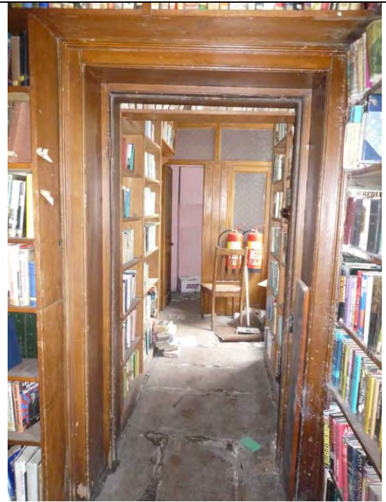
Fig.52: Missing door leaf to opening giving access from G15 to G16.
