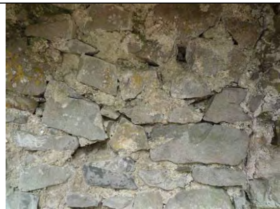
Fig.42: Open-joints to northern boundary wall.
