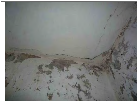
Fig.47: Cracking of ceiling plasterwork to G10.
