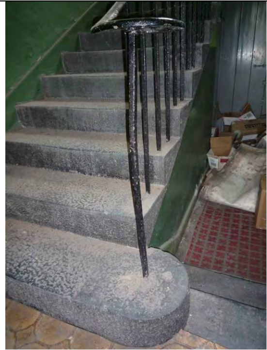
Fig.56: Missing wrought-iron balusters newel post of staircase to G11.
