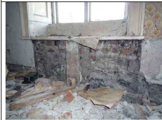
Fig.53: Missing apron panel to window opening at F07.
