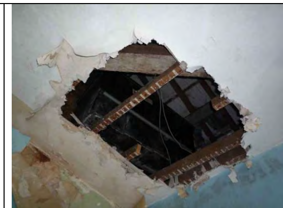
Fig.48: Significant hole in ceiling plaster over F01.
