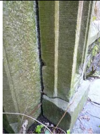
Fig.24: Significant open-joints to the door surround of the east elevation.
