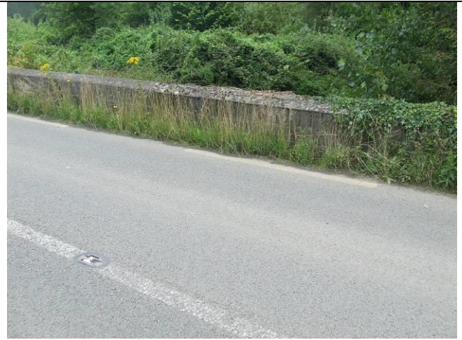
Plate 7: Showing concrete block rebuilt section of northeast elevation of bridge (AH07), facing north.
