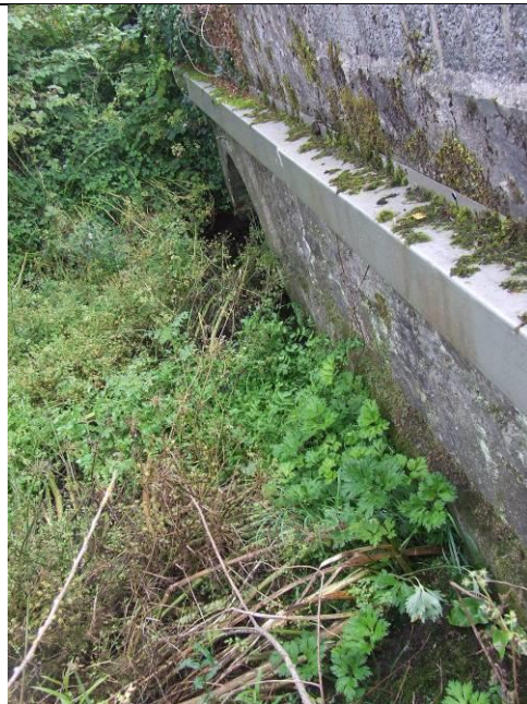
Plate 6: Showing southern arch and northeast elevation of bridge AH07, also showing concrete block upper section, facing south.
