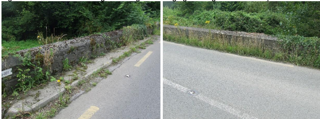
Figure 21: South parapet wall and Figure 22: rebuilt northern parapet wall
