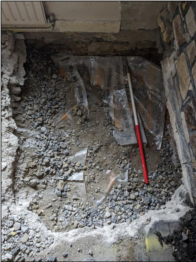
Plate 5 Mid-ex of Test Trench 3 in building No 6 showing hard fill and plastic damp proof membrane.
