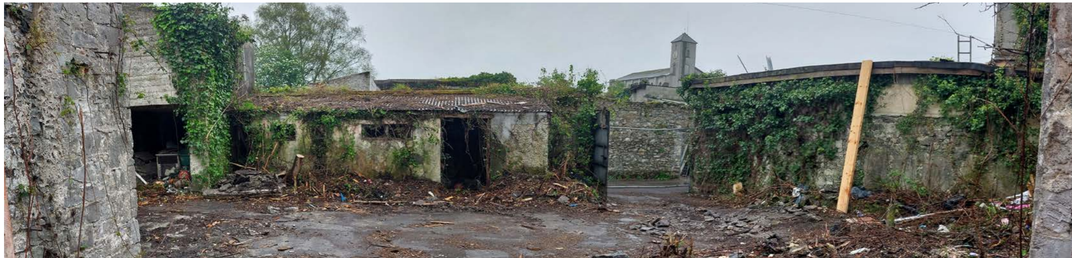
18 - PANORAMA AFTER VEGETATION CLEAR OUT SHOWING REAR CONCRETE SHEDS TO BE DEMOLISHED
