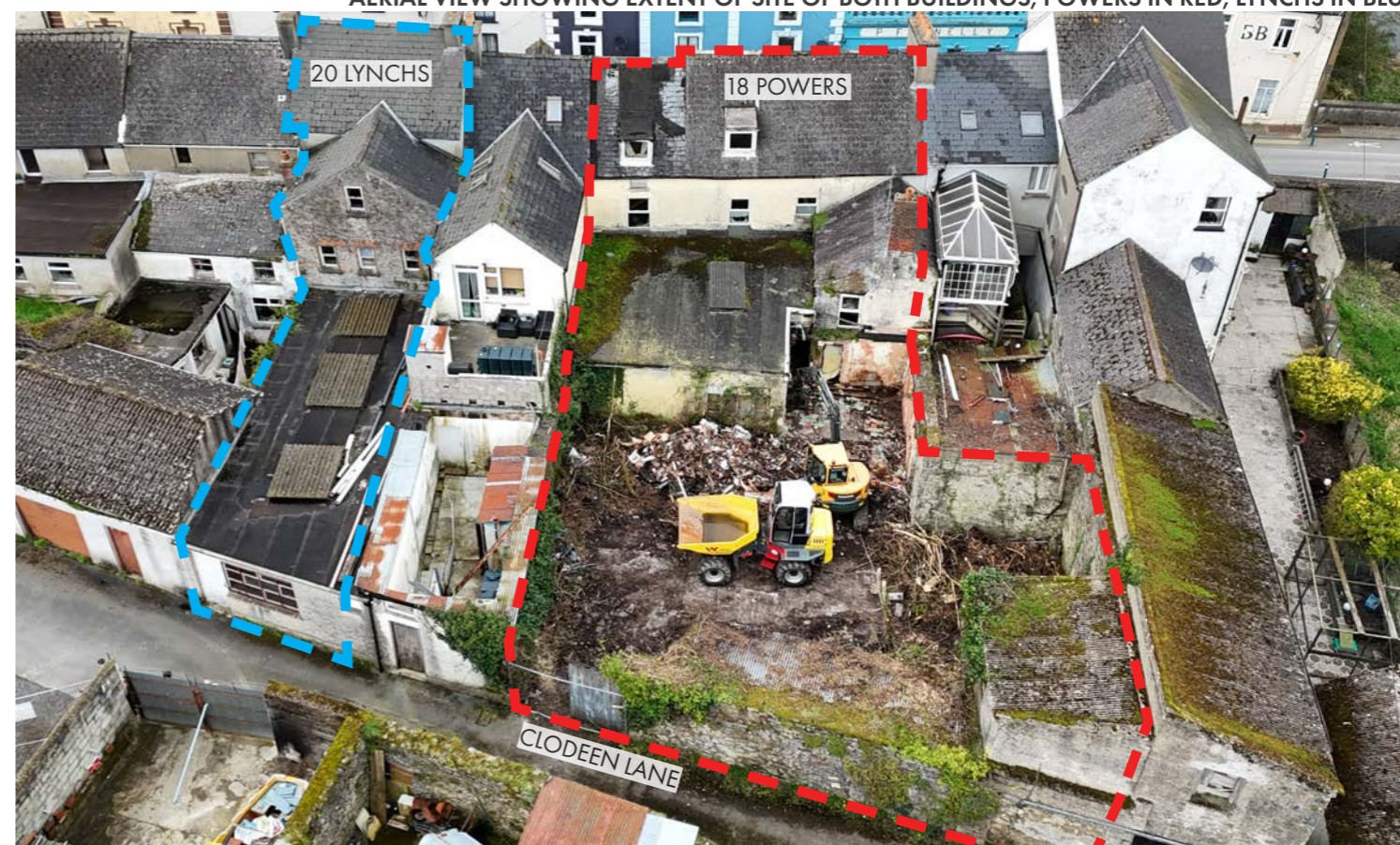
AERIAL VIEW FROM REAR SHOWING EXTENT OF SITE OF BOTH BUILDINGS, POWERS IN RED, LYNCHS IN BLUE
