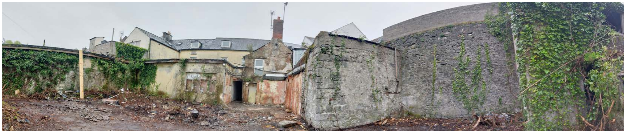
18 - PANORAMA AFTER VEGETATION CLEAR OUT SHOWING SINGLE STOREY EXTENSION TO BE DEMOLISHED
