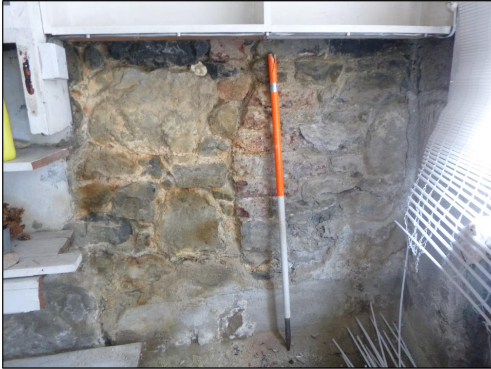
Plate 9 Ground floor S party wall to No. 20 showing extension or rebuild of street frontage (Source: Shanarc Archaeology Ltd. 10.04.2024).
