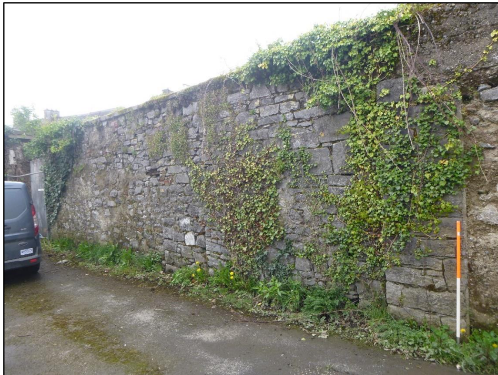
Plate 5 No. 18 boundary to rear on Clodeen Lane displaying infilling and rebuilding to limestone wall (Source: Shanarc Archaeology Ltd. 10.04.2024).
