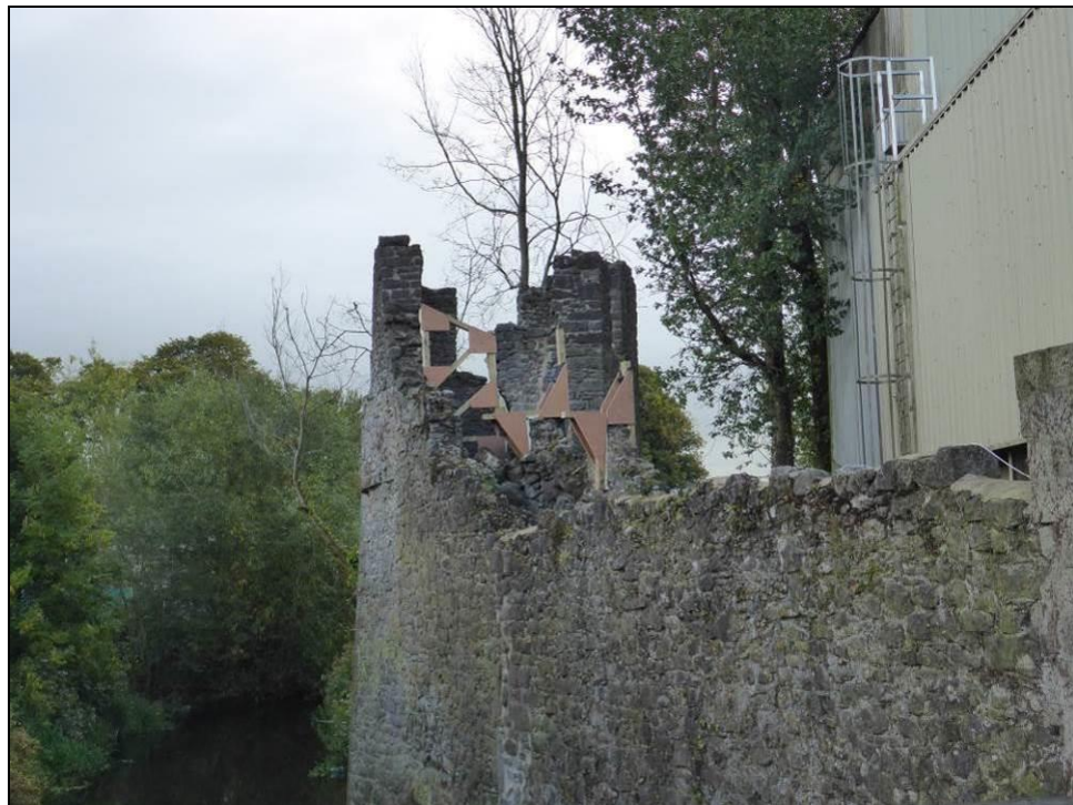
Plate 21 Evan's Tower and wall walk vegetation removed and bracing in place September 2015
