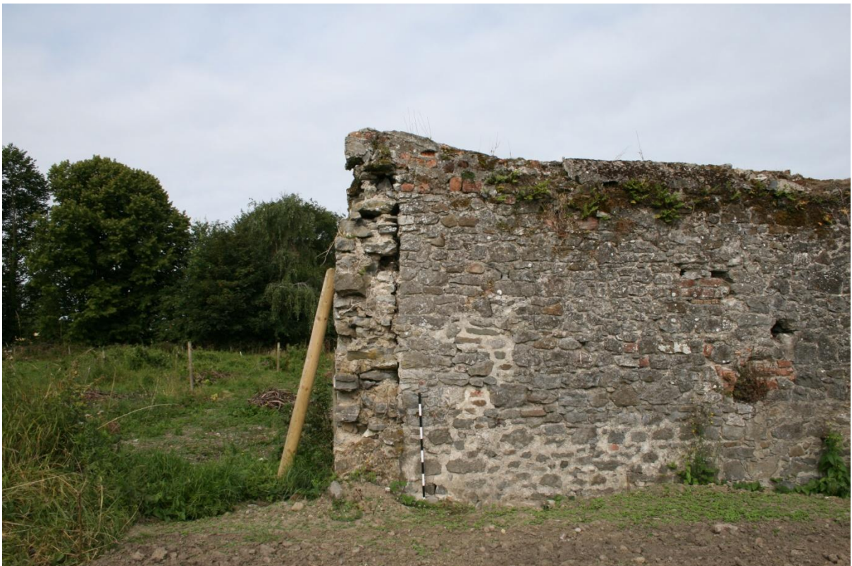
Figure 12: Remnant of earlier wall abutted by walled garden walls, for south-west range of former house complex, from east.
