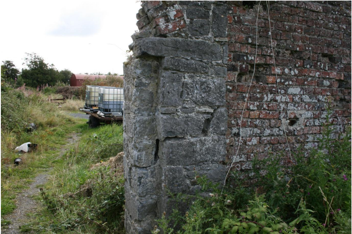
Figure 23: Large crack in south pier of cart entrance.
