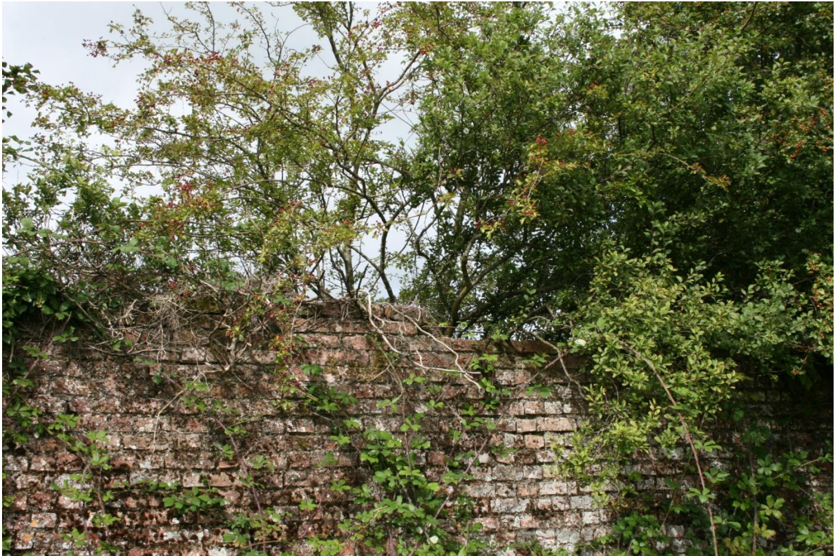
Figure 42: Loss of stone and brick from wall head, west wall.
