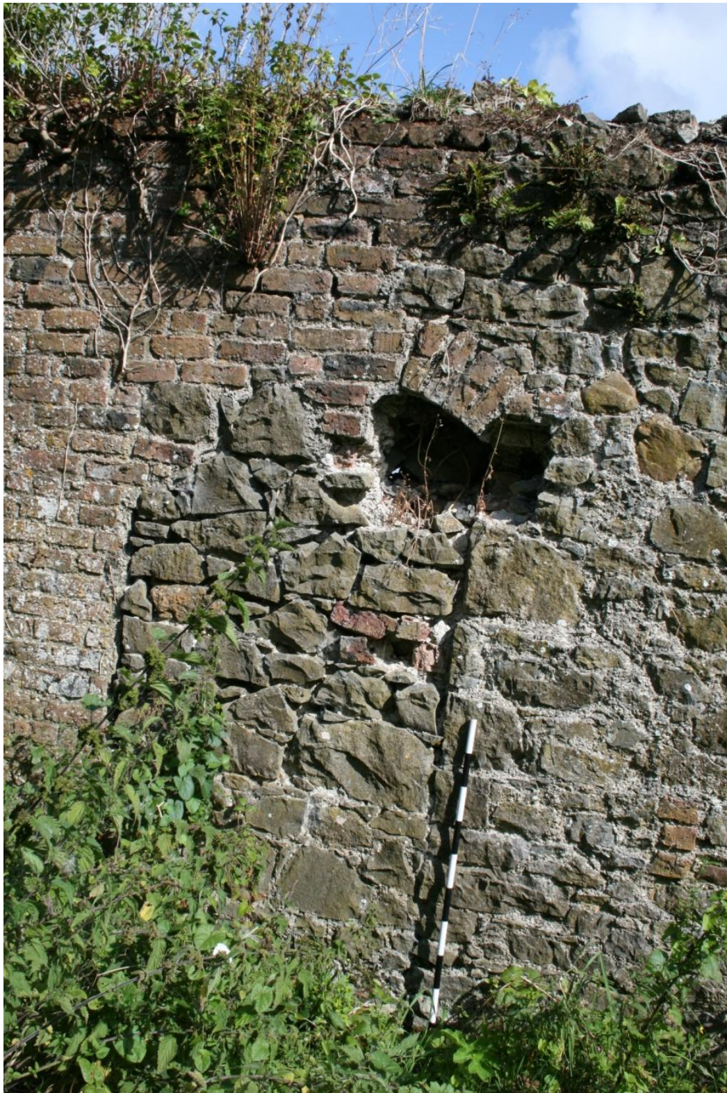
Figure 32: Blocked pedestrian entrance to walled garden at south -west of south wall.
