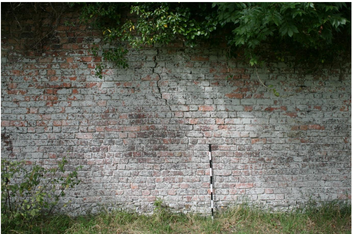
Figure 43: Crack in west wall, probably caused by tree growth on opposite side of wall.
