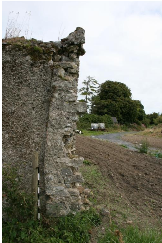
Figure 13: Remnant of earlier wall with quoins abutted by walled garden walls, for south-west range of former house complex, from south.
