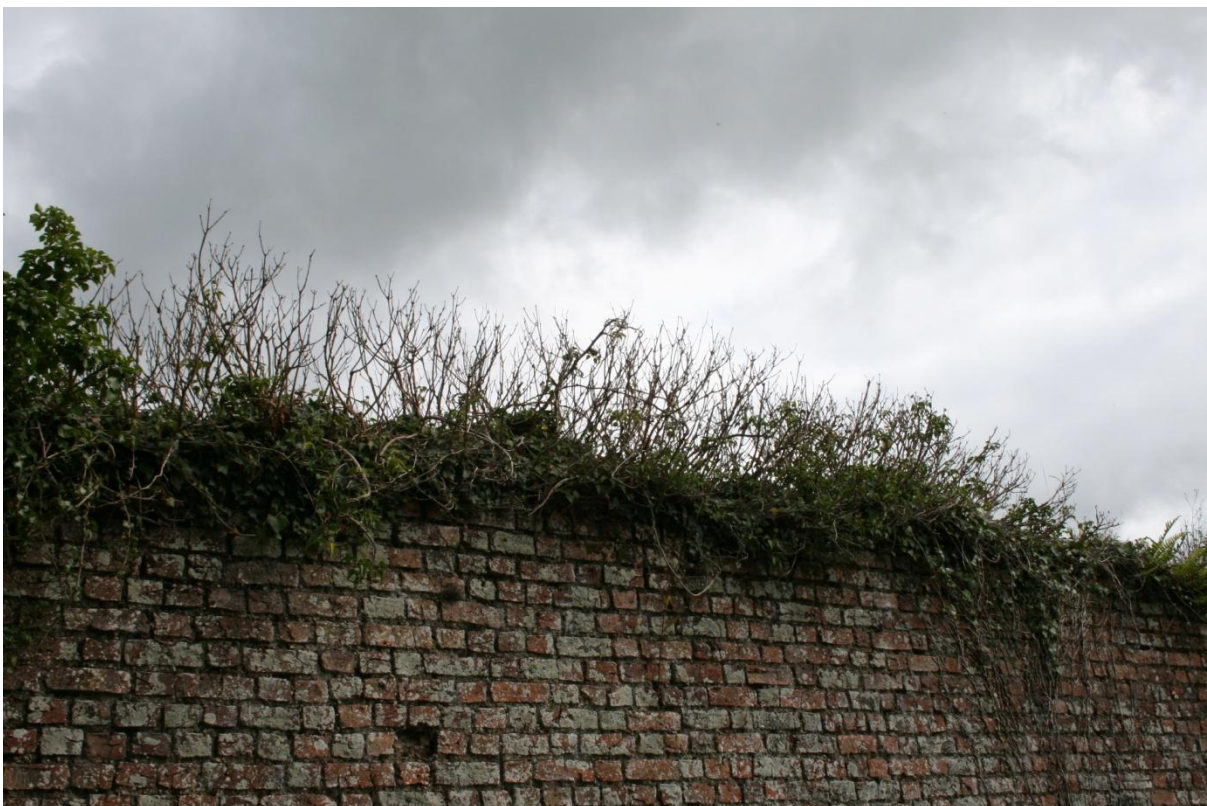
Figure 45: Growth on top of wall head, south wall.
