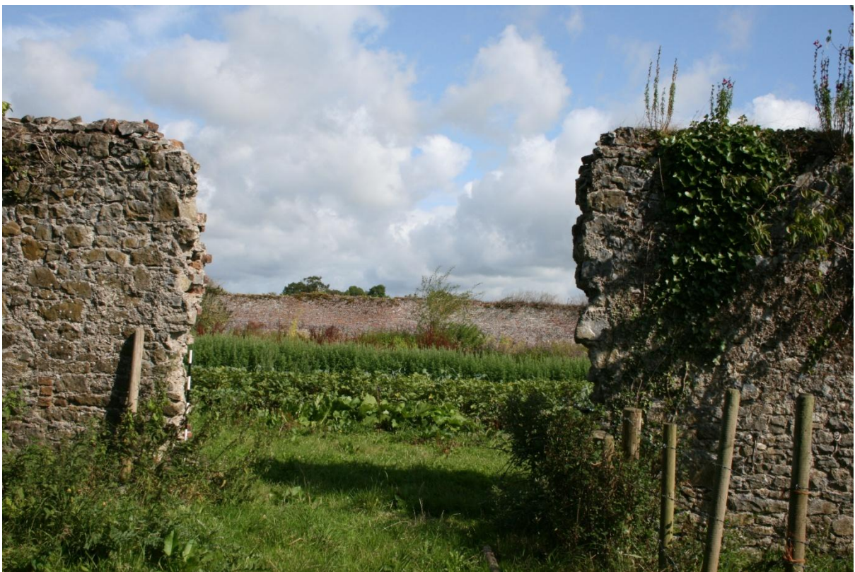
Figure 31: Large ope broken through south wall.
