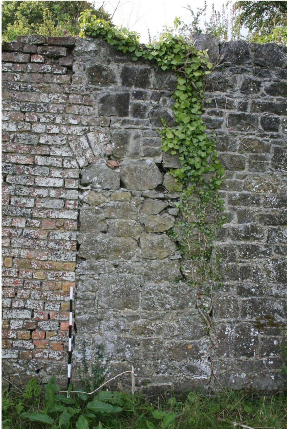
Figure 37: Blocked pedestrian entrance door south wall interior. Note stone repair to brick wall.
