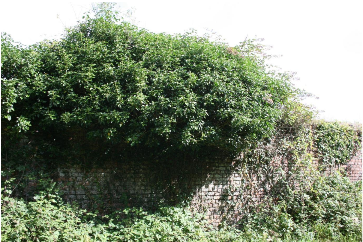
Figure 36: Extensive ivy growth on top of south wall.
