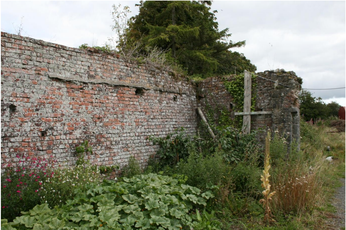
Figure 53: Joist holes from former lean-to, south wall interior, east side.
