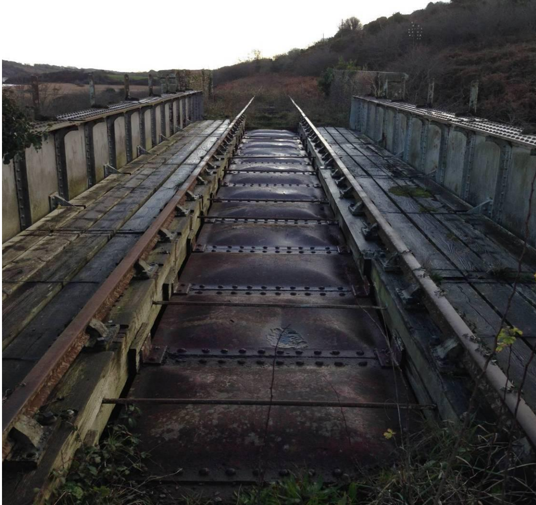
Photo 4.14: Masonry/Iron Under-bridge over Glenmore River located in cSAC (IR Ref UBJ 441) Ch 13+800
