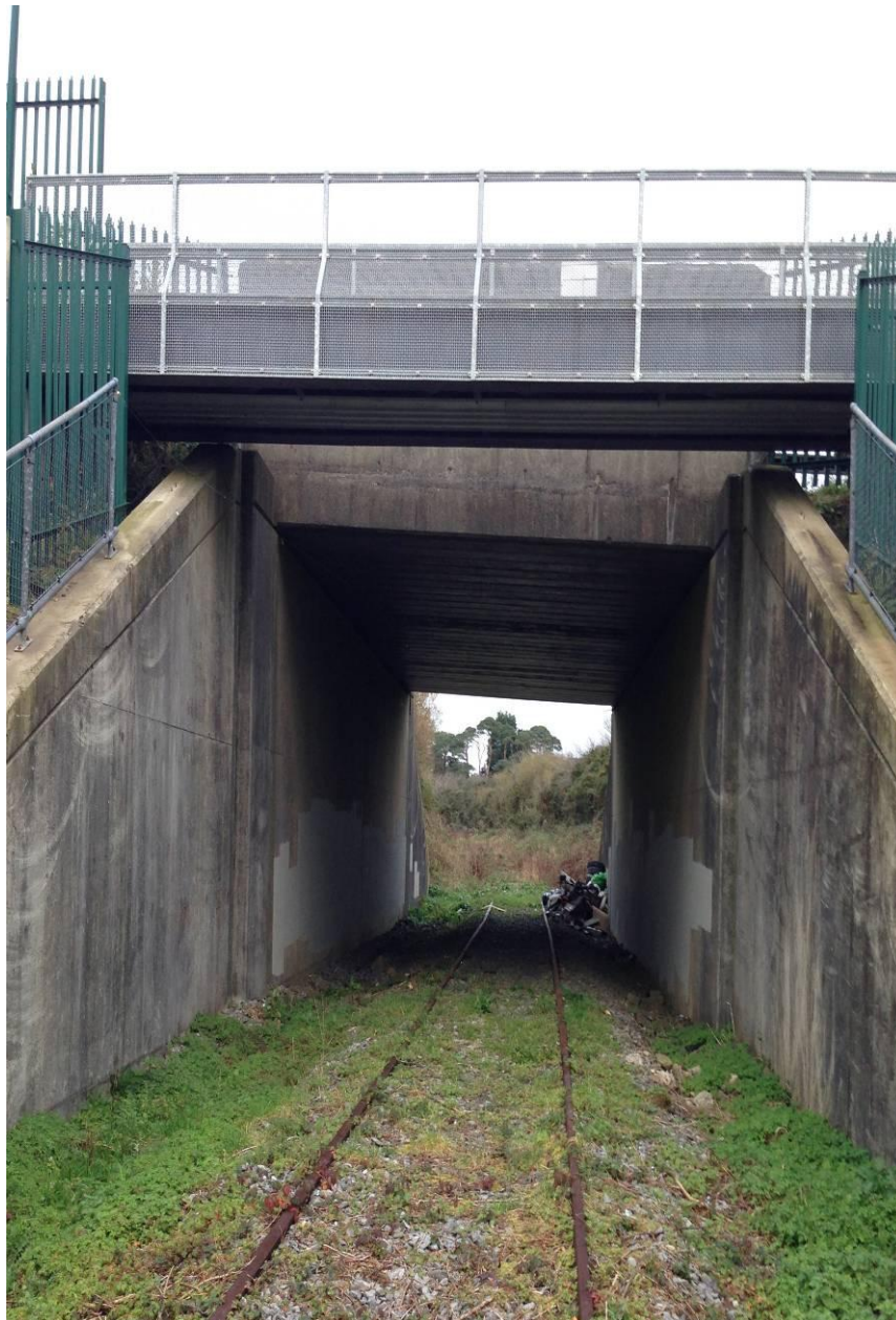
Photo 4.3: Looking north under the N29 Concrete bridge IR Ref: OBJ 461A (Ch. 3+600)
