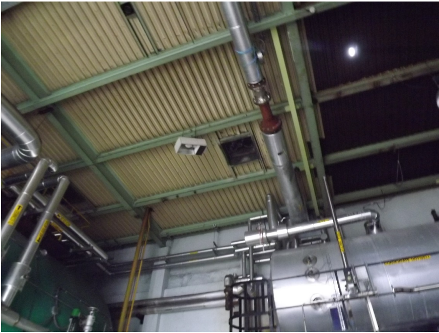
Interior view of the phase 3 of the Brewhouse Showing the vats and the colour coding of the green beams
