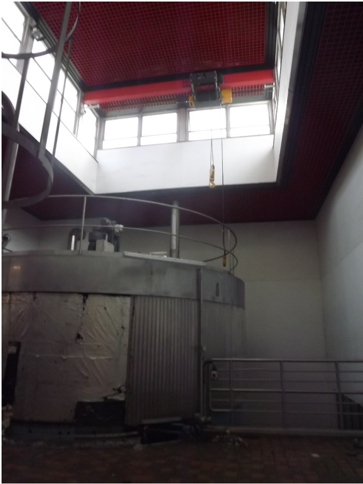
Interior view of the phase 3 of the Brewhouse The roof light is designed as an 'extended plane of the flat roof' pushed upward The light comes in from the side. This should be reinstated
