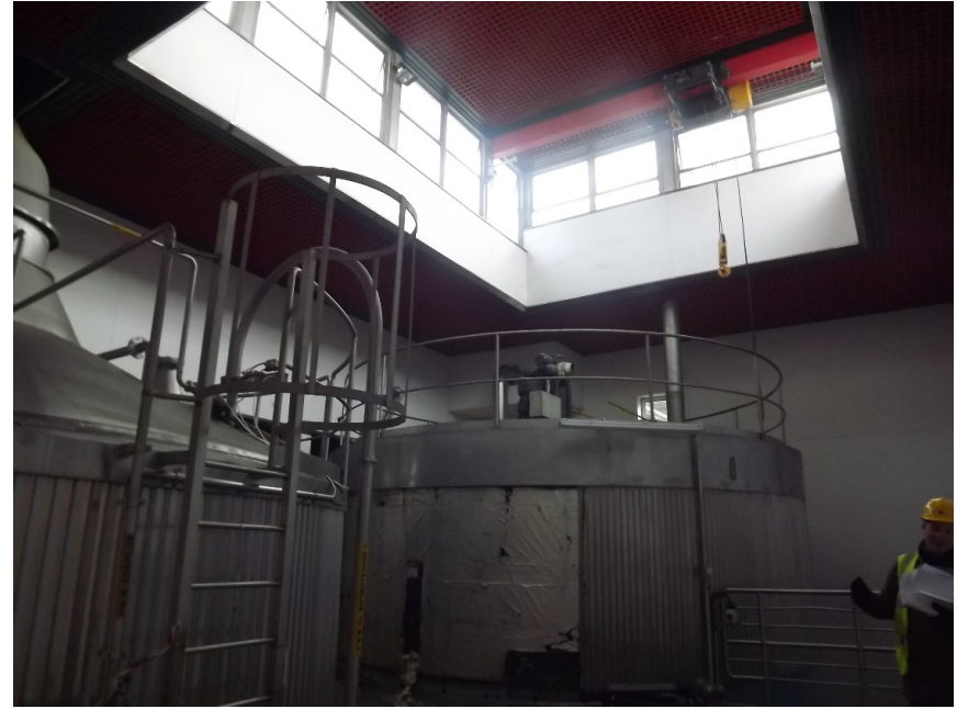
Clerestory windows of the rooflight in the central block phase 3 over the central vats. The rooflight is designed as an 'extended plane of the flat roof' pushed upward. The light comes in from the side. The exterior lines of this rooflight have been distorted as it has been reclad in bulky cladding.
