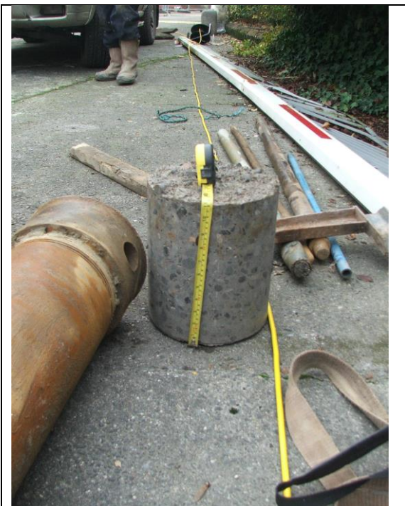
Plate 13 Showing depth of reinforced concrete in yard to west of Brewhouse Building, from geotechnical sampling under Ministerial Consent C00773.
