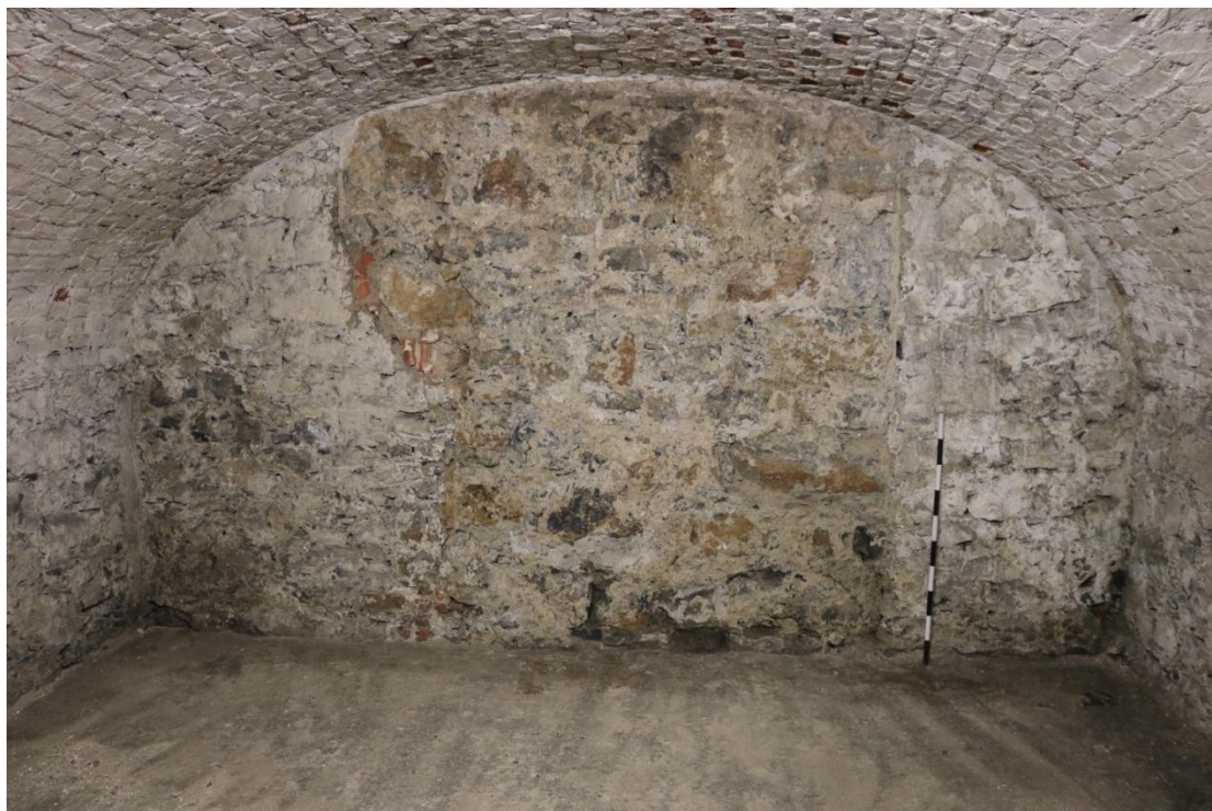
Figure 69: The east wall of the basement in the centre room, showing the wall 159 flanked by the blocking walls 161 and 162, from the west
