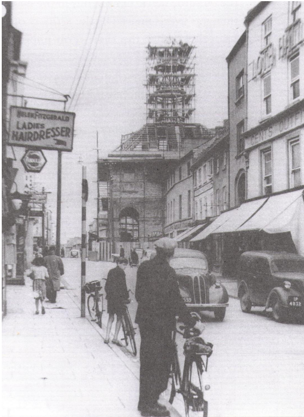
Figure 34: Building works underway c. 1953 at the Tholsel, from south (reproduced from Bradley, Discover Kilkenny, p. 63)
