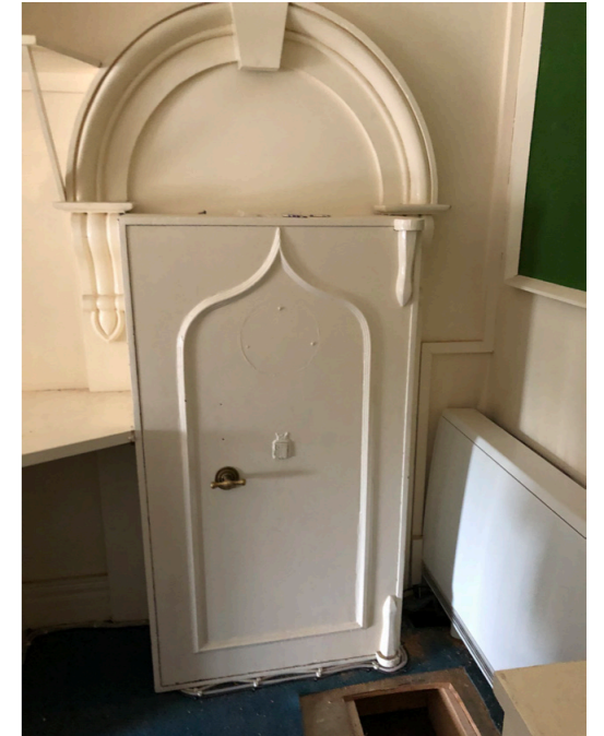
Third floor: Suspected window surround
