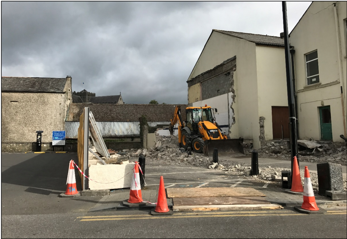
Plate 4: Monitoring demolition works at the west end of the Mayfair Building, June 2017
