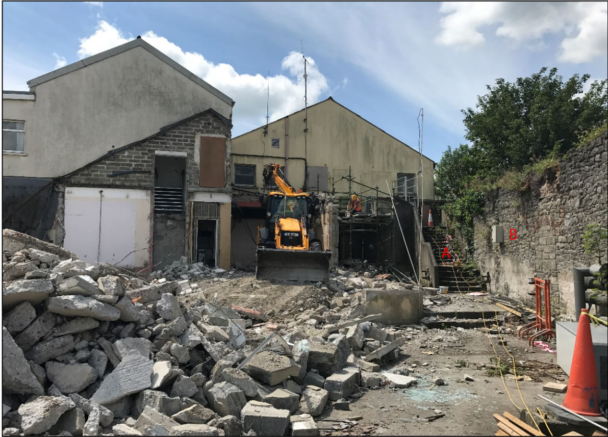
Plate 3: Demolition of eastern portions of the Mayfair Building adjacent to the city wall, looking west in 2017. Note the boiler house and concrete steps remaining in situ (A), and the vibration monitor fixed to the wall (B).
