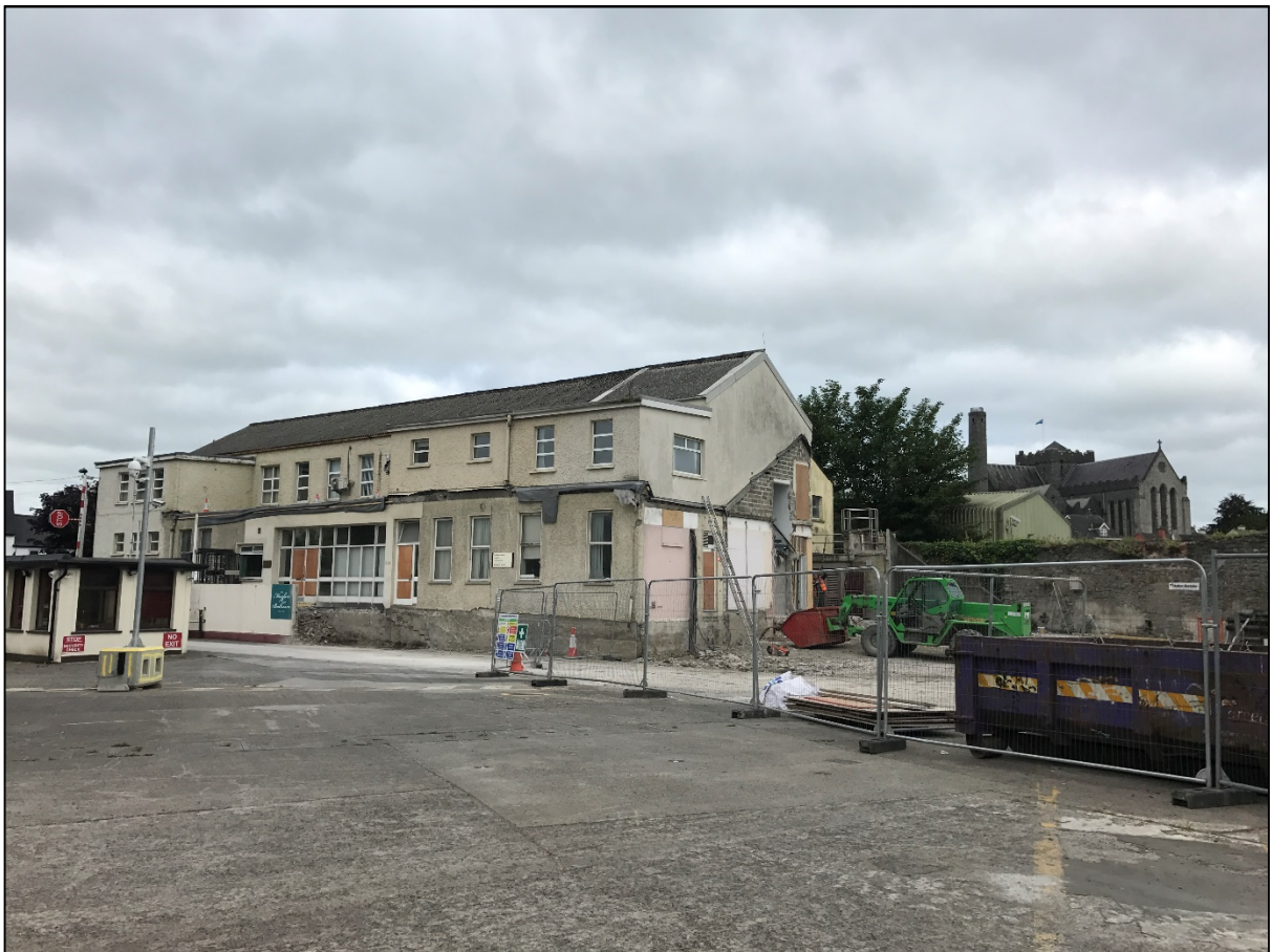
Plate 2: Mayfair during demolition of modern portions at the east end of the building in 2017
