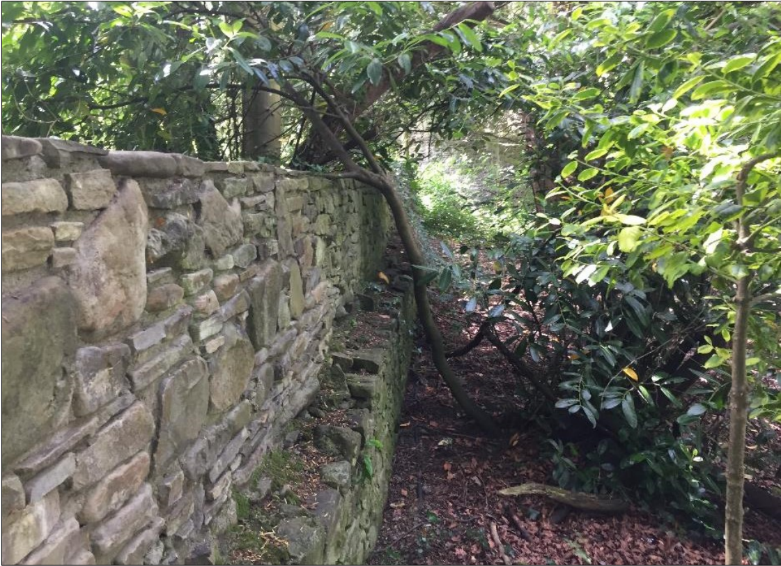
Plate 31: Modern (c.2000) stone masonry on top of older lower portion of riverside wall on west bank of Dineen River extending to abut north elevation of west abutment of bridge through vegetation to centre of photograph.
