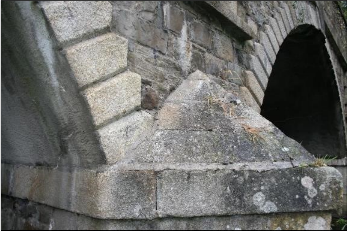
Plate 23: Detail of downstream cutwater cap (on south elevation). Inappropriate cement pointing here and over all elevations poses a long-term risk to the proper performance of masonry.
