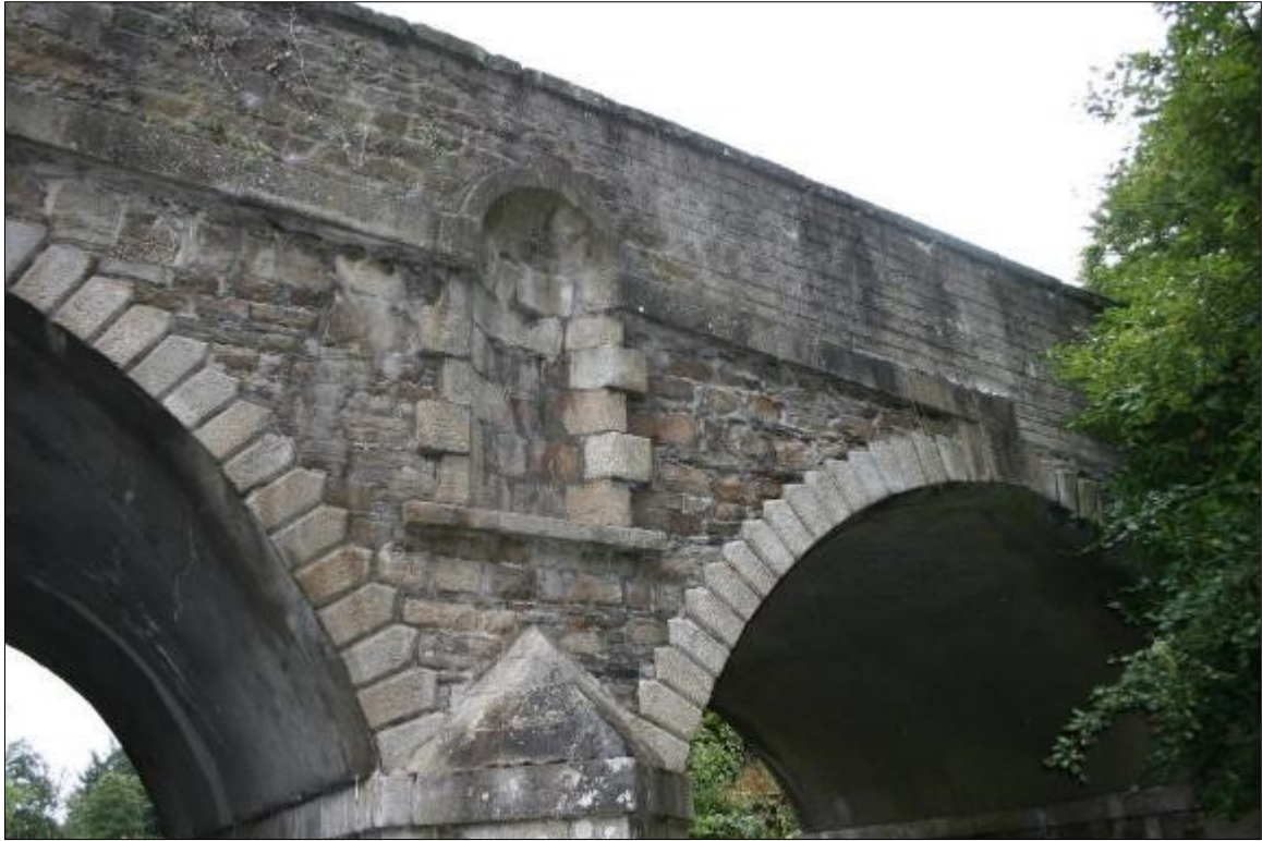
Plate 21: Detail of spandrel over 2 nd pier from east abutment. Parapet here was partially reconstructed with concrete blocks sometime within last 30 years
