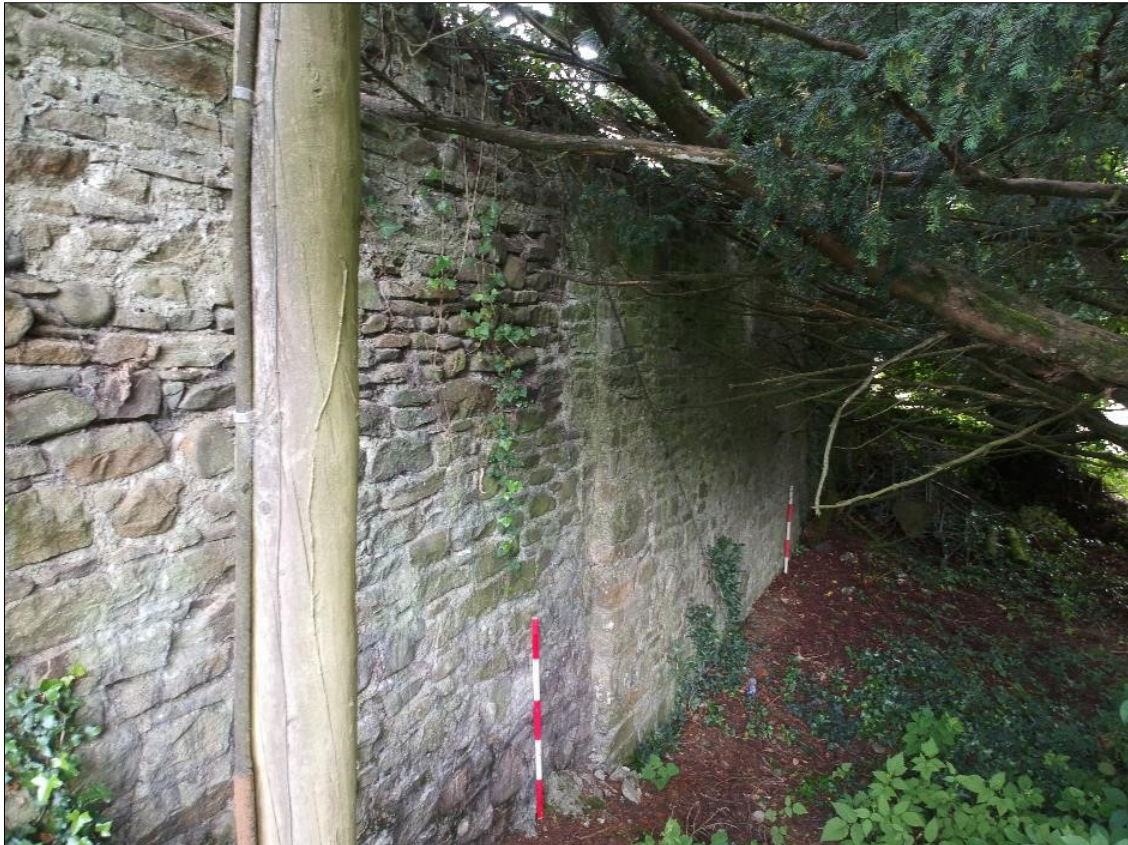
Plate 30: North elevation of west abutment with small step visible in wall just right of ranging rod. No evidence of a structure having existed here (such as joist sockets)
