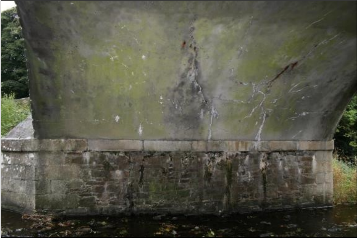
Plate 17: West shoulder of arch soffit within 2 nd arch from west abutment. Limited moisture ingress from bridge deck is escaping through pier masonry and also through cracks in gunited arch soffit.
