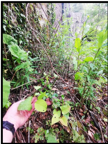
Plate 4: Two small Japanese knotweed plants close to the foundation wall of the N78 bridge near Castlecomer in May 2019.
