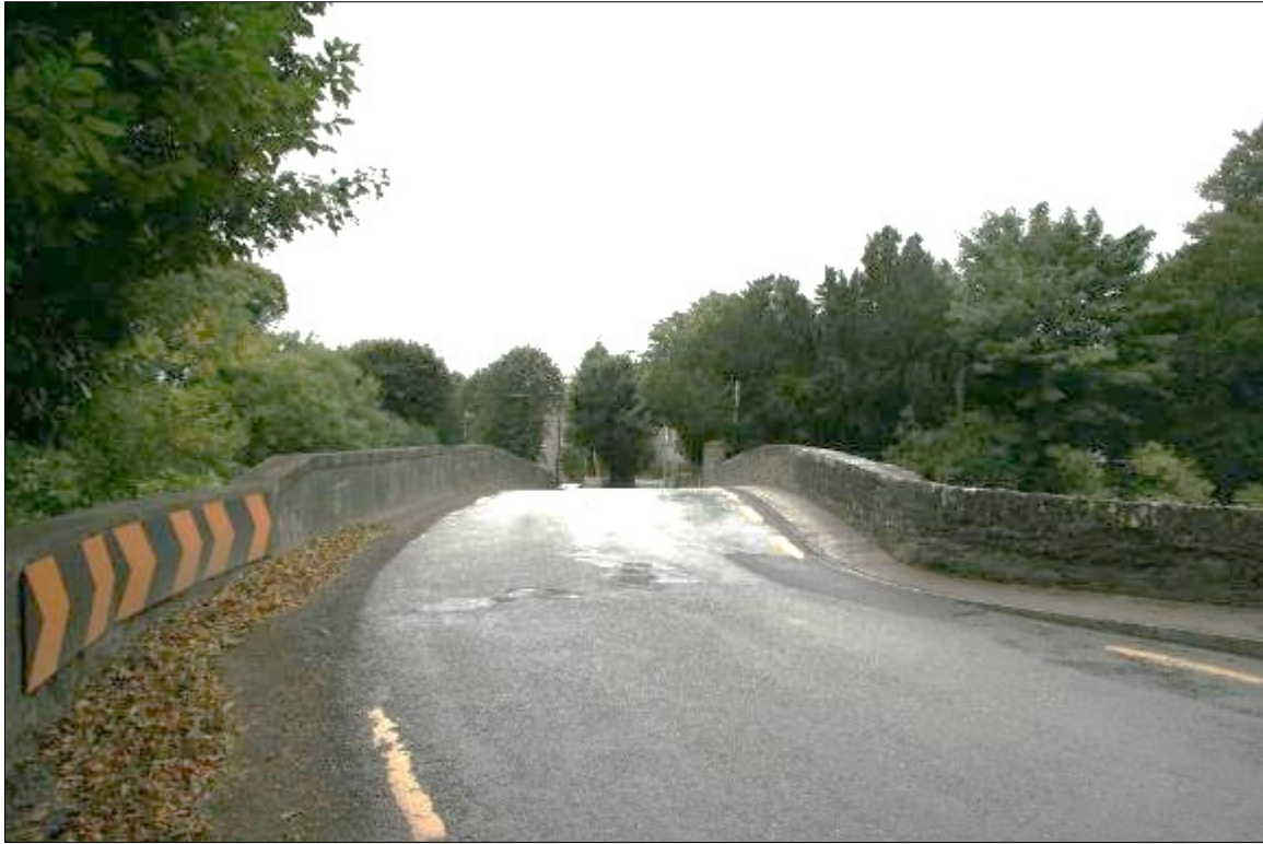
Plate 5: Approach to bridge from east with some ongoing damage to deck surface above springing point above east-most pier.
