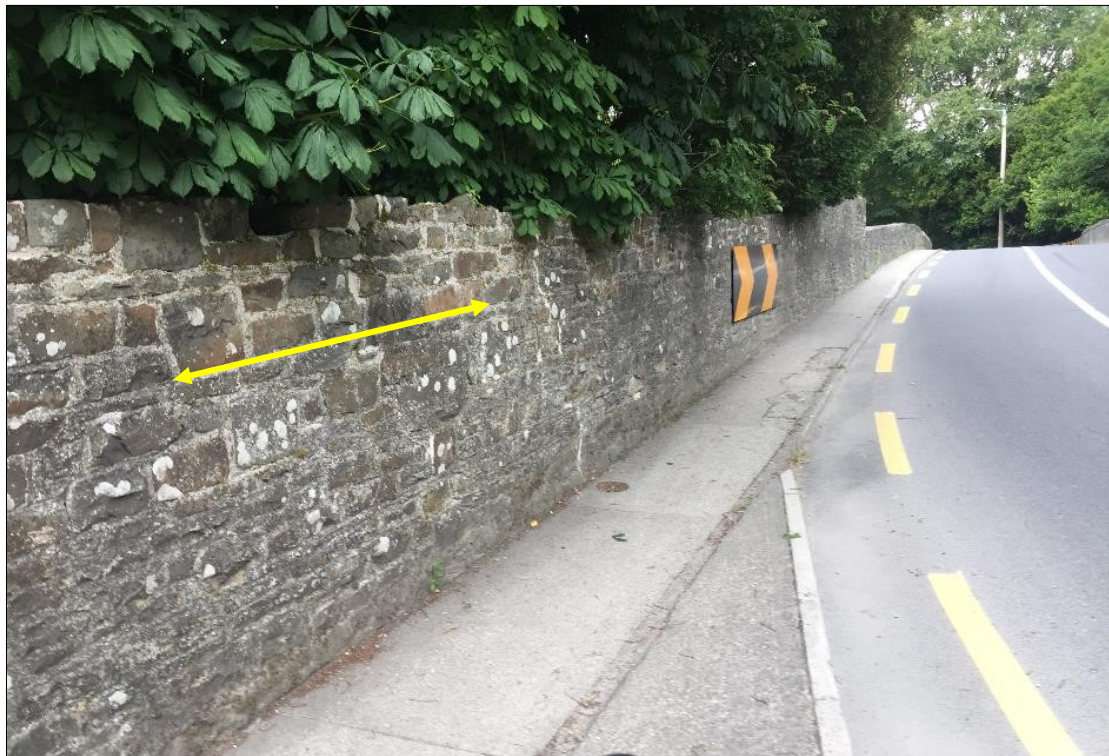
Plate 26: View of the north approach wall to west abutment of the bridge. Masonry above arrowed line appears to be more modern with more face-bedded stones and longer vertical joints than historic masonry below. This is most likely to have been the result of raising the original approach wall to the bridge in the last 100 years to provide privacy to the garden of La Rive.
