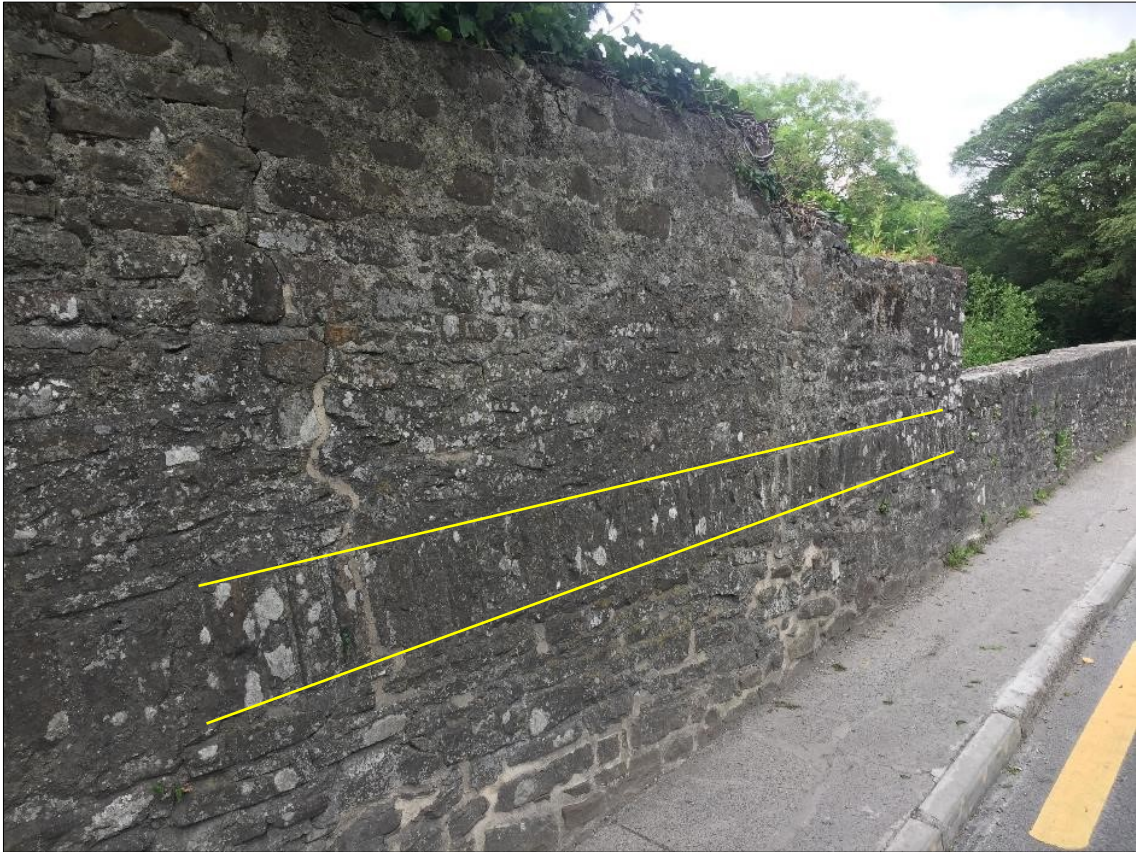
Plate 27: Original approach parapet to north-west abutment with original low-level course of vertical coping stones (highlighted by the yellow lines) surmounted with random sandstone rubble wall.
