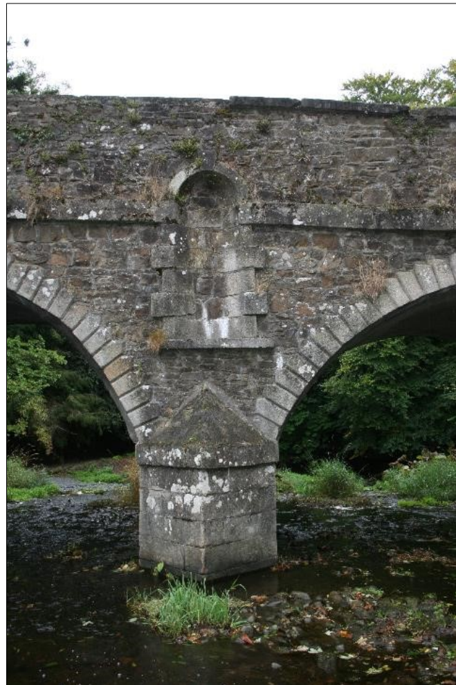
Plate 14: Detail of north elevation of spandrel and 2 nd pier from west abutment
