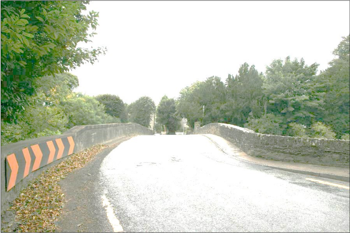
Plate 5: Approach to bridge from east with some ongoing damage to deck surface above springing point above east-most pier.
