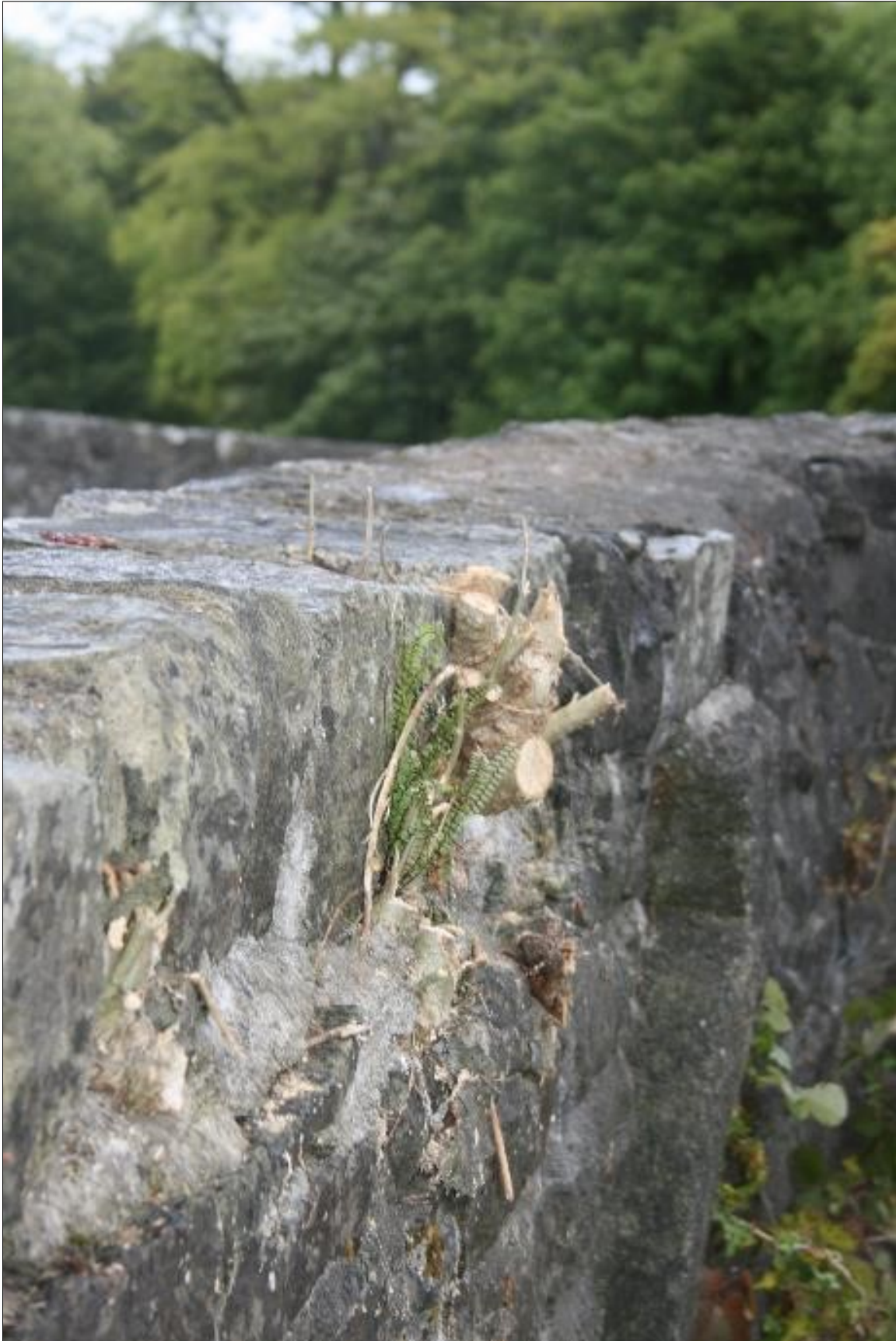
Plate 7: Localised deep-rooting vegetation on parapet exterior being kept trimmed back to restrict its development until it can be fully removed and affected masonry repaired.
