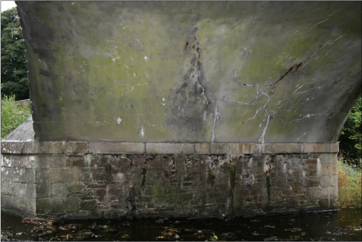
Plate 17: West shoulder of arch soffit within 2 nd arch from west abutment. Limited moisture ingress from bridge deck is escaping through pier masonry and also through cracks in gunited arch soffit.
