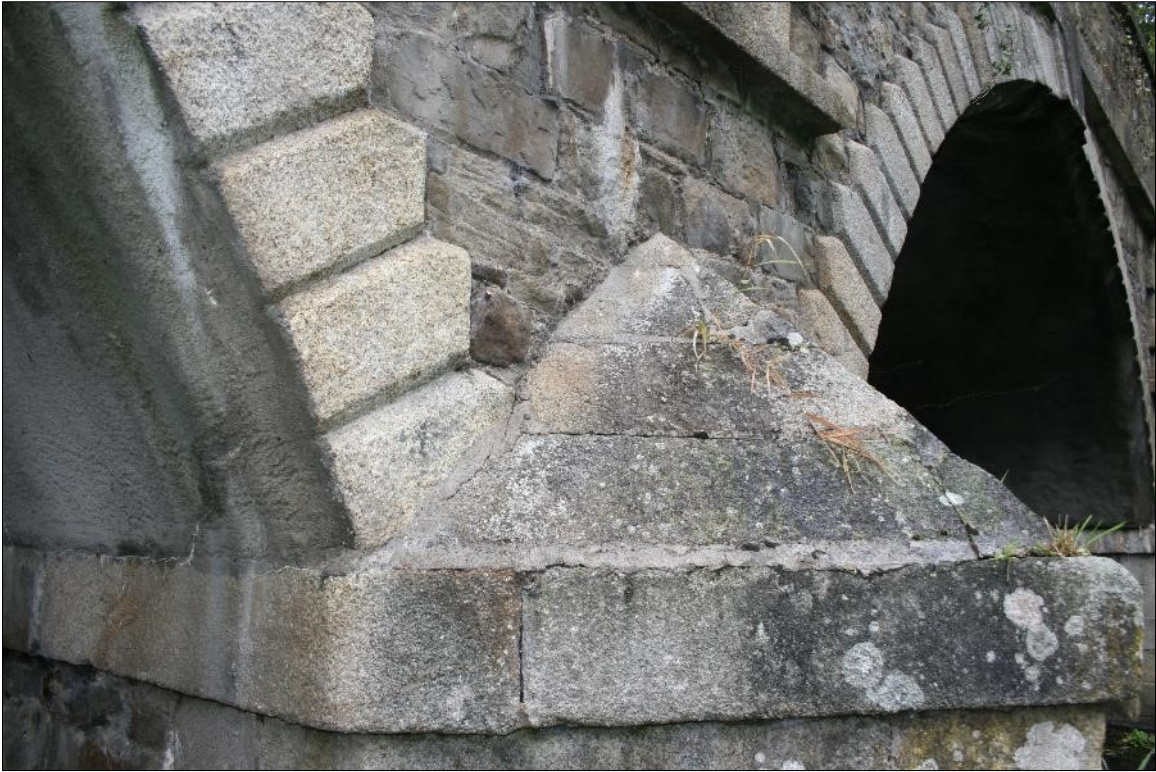
Plate 23: Detail of downstream cutwater cap (on south elevation). Inappropriate cement pointing here and over all elevations poses a long-term risk to the proper performance of masonry.
