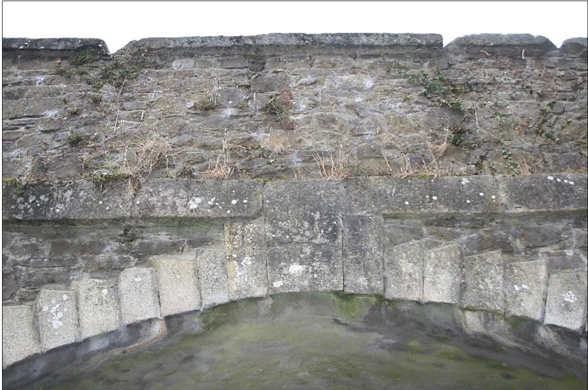
Plate 15: Keystone, voussoirs, string course and exterior parapet detail over 2 nd arch from west abutment
