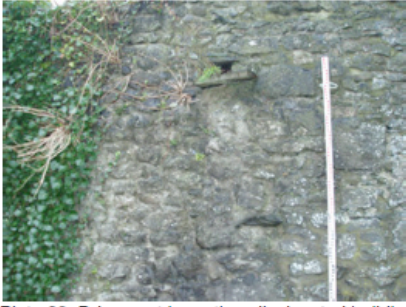
Plate 23. Drip spout in north wall, claustral building.
