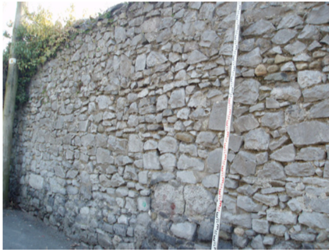
Plate 10. Boundary wall showing at least three phases of building. Upper and middle build are 19th century, lower wall F12 is probably 18th century in date.
