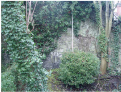
Plate 36. Scar of steeply pitched gable in plaster visible in western boundary wall.
