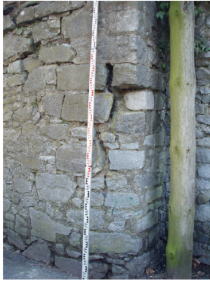
Plate 9. Chamfered corner and quoins of barracks. Masonry as in boundary wall F12.
