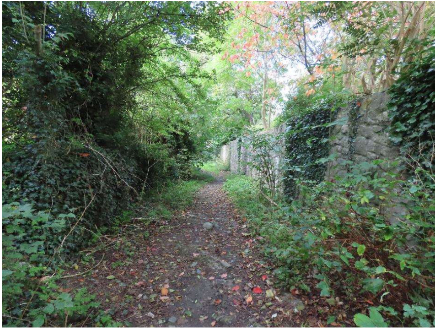
Photo 3 – high stone wall to rear of Hotel Kilkenny running along northern boundary of lane is very well pointed and has no potential for roosting bats
