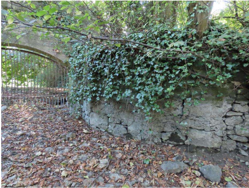
Photo 9 – fissures in wall on northern side of old ford – no potential for bats Habitats present – BL1 (Stonewalls and other stonework)
