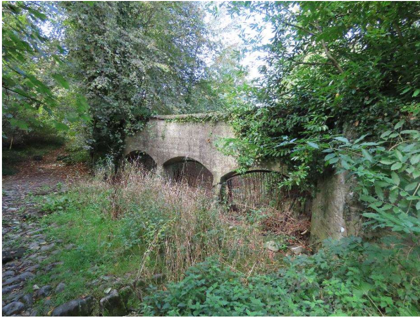
Photo 5 – upstream (southern) elevation of former bridge structure on Cootes Lane Habitats present – BL3 (Buildings and artificial surfaces) – concrete wall of ford
