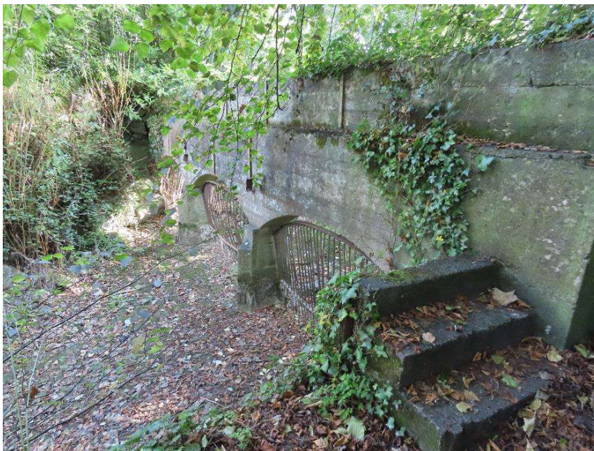
Photo 8 – northern (downstream) elevation of old ford – this structure was surveyed as assessed as having no potential as a bat roosting site
