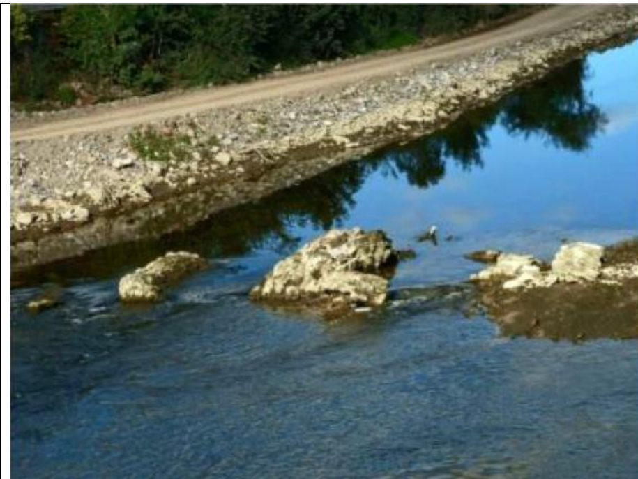
Plate 6 Image of haul road for Kilkenny Flood Relief Scheme on west bank of River Nore at location of proposed River Nore Pedestrian and Cycle Link Project. Note abutments of Greensbridge AH03 in river (courtesy OFW).
