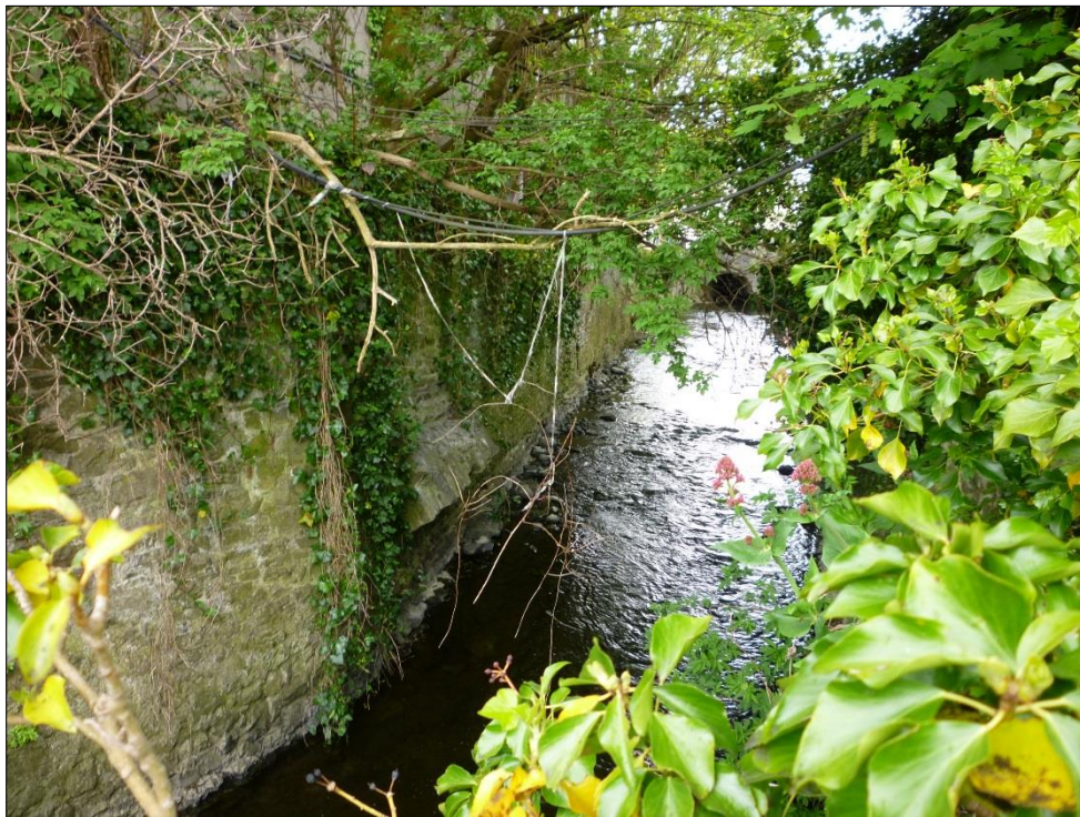
Plate 75 City Wall to the rear of the Mayfair Building taken from the east showing spring stones of a former bridge site
