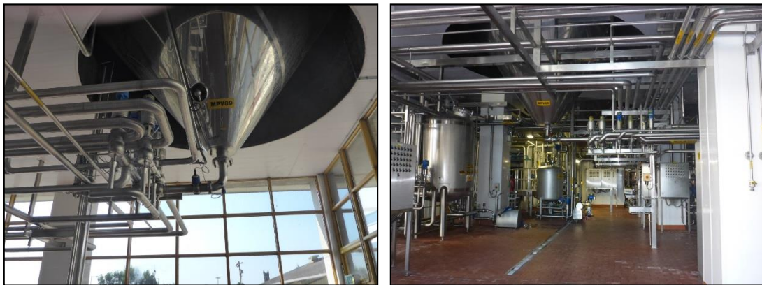
Plates 63-64 Maturation Building internal workings
